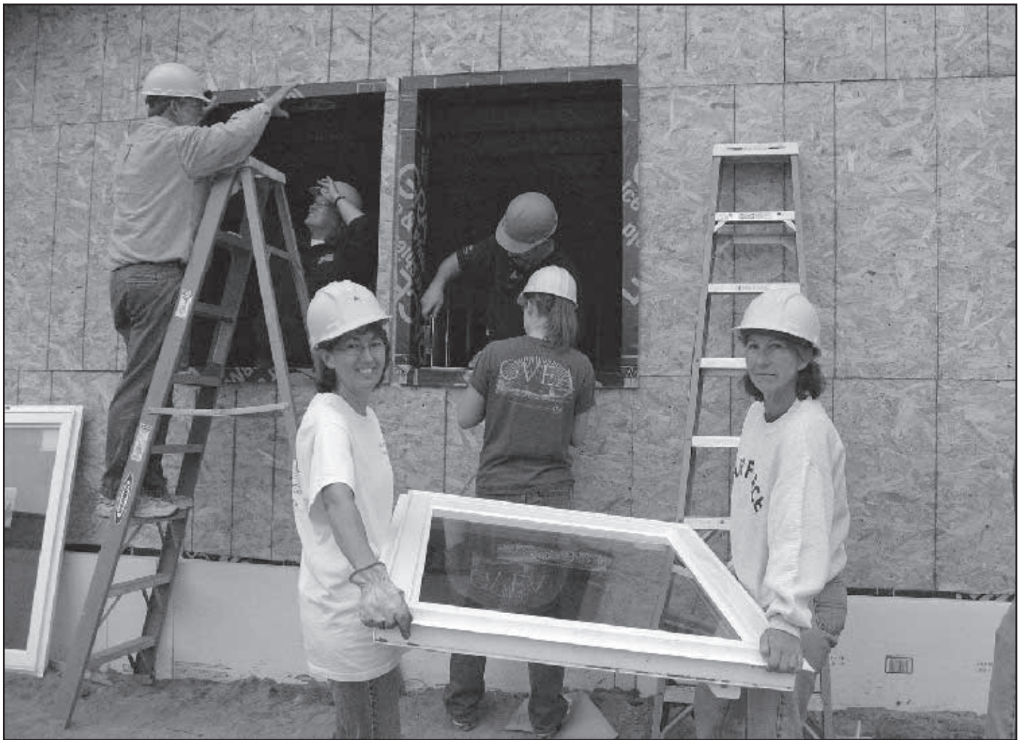
A team from Golden Valley Electric Association in Fairbanks, Alaska, installs windows at a Habitat for Humanity home.
